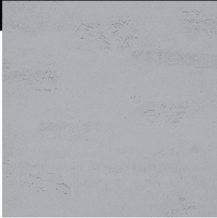
MOA-##-S | Pitted Surface
